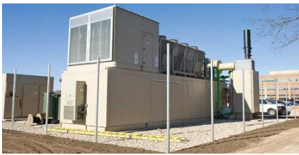
Engine/generator set with heat recovery and gas clean up
