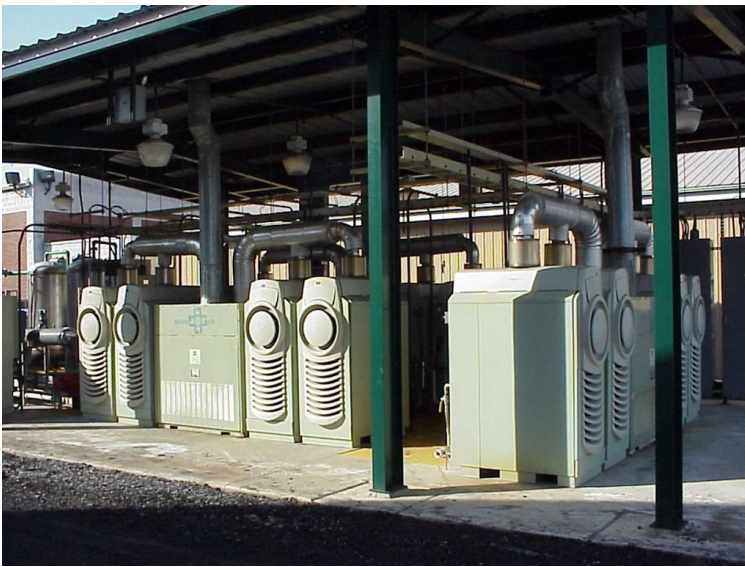
The CHP plant is housed under a 1,000 ft 2 pavilion
