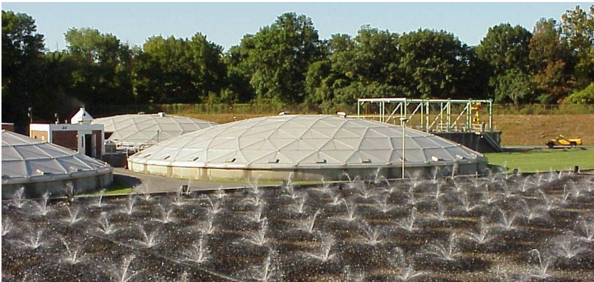
A view of the rock media trickling filter (foreground) and various settling tanks (background)
