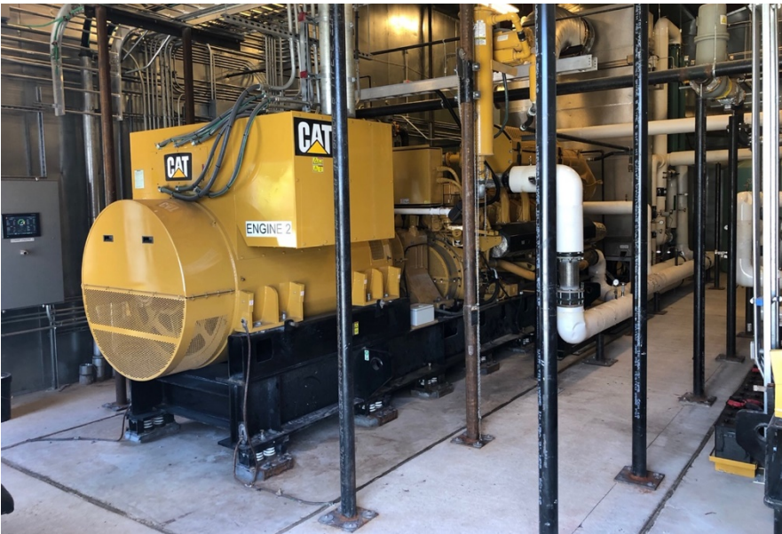
Two Caterpillar – 2,485 kW Engine Generators Systems in CHP Plant
