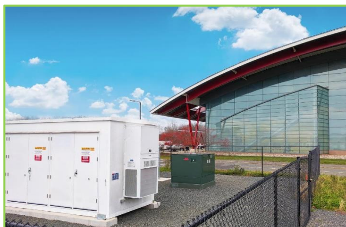
Battery storage project near the central heating plant
