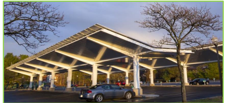
Solar canopy project at the central heating plant
