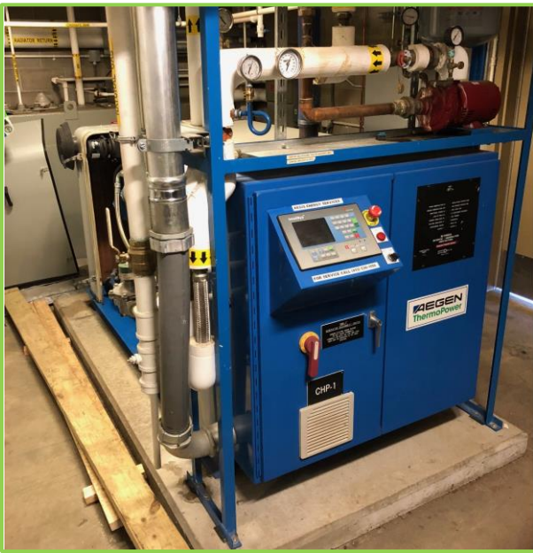
Aegis 75 kW CHP system including a reciprocating engine and induction generator.
