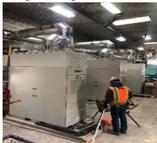
IMAGE COURTESY OF HORIZON POWER SYSTEMS
