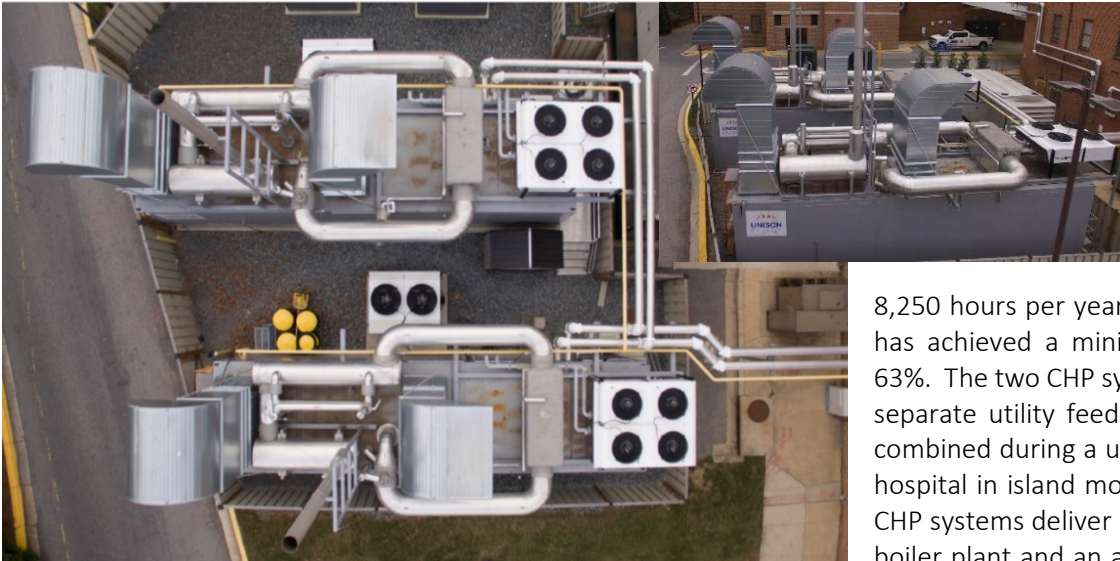
Two 2G Energy – 600 kW Packaged CHP Systems
