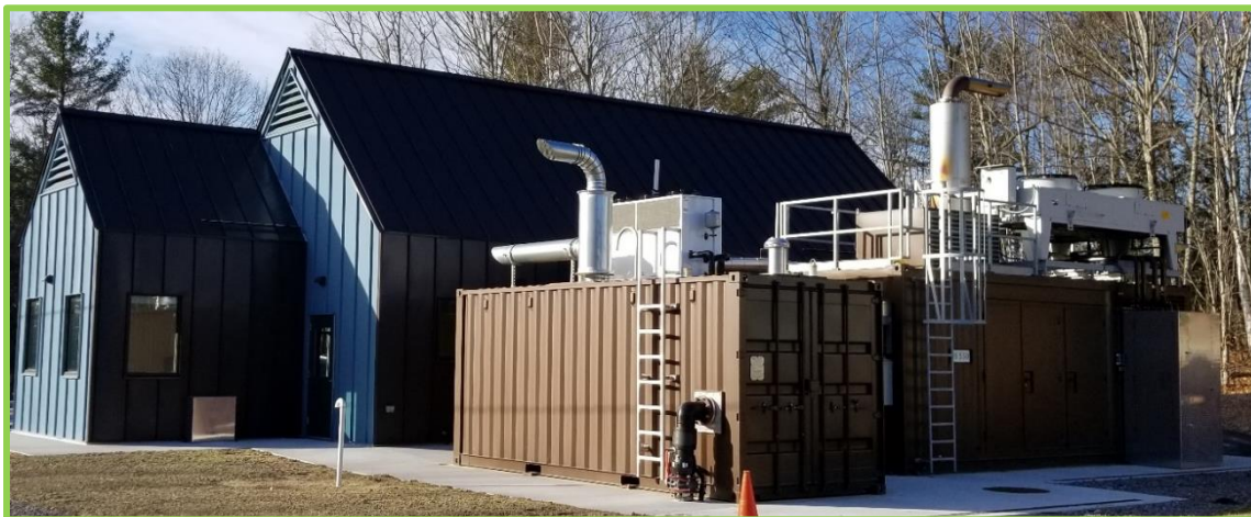
Hatch Hill Landfill's CHP system, dehydration skid, and operations facility
