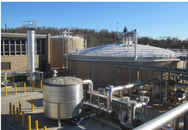
Anaerobic Digester and Gas Cleaning Equipment Photo Courtesy of City of Springfield
