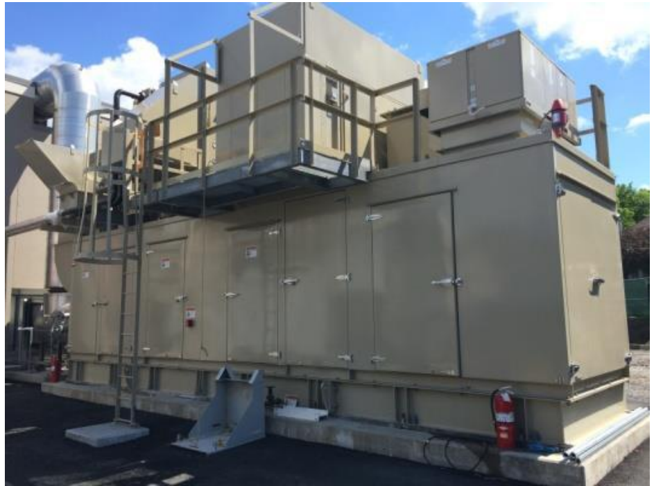
Outdoor Enclosure of Kawasaki GPB17D gas turbine at Union College
