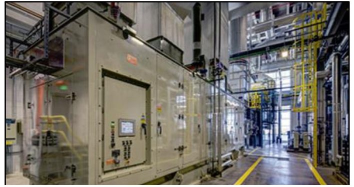
Enclosure for 5.7 MW Solar Taurus Gas Turbine with 50,000 lbs/hour Heat Recovery Steam Generator
