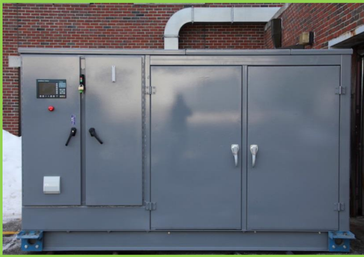
150 kW CHP system prior to installation at St. Mary's d'Youville Pavilion, a non-profit nursing home.
