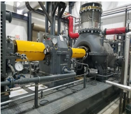
Adkins Plant, Backpressure Steam Turbo-Generator Set
