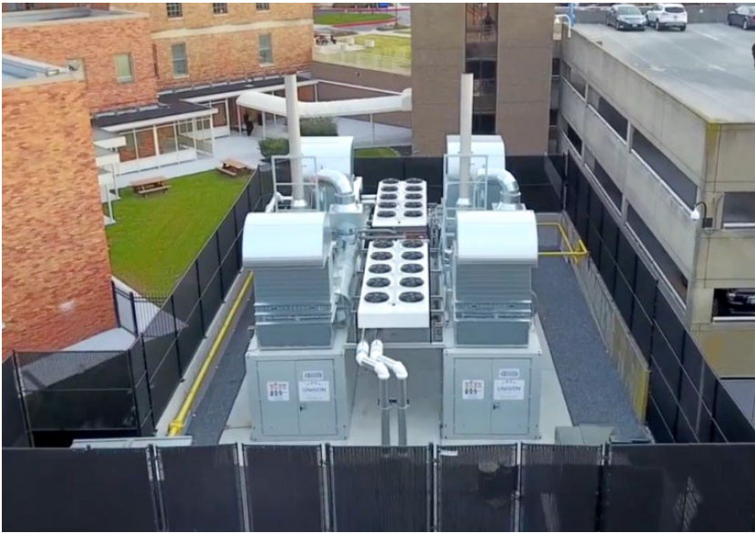
Two 2G Energy – 1.56 MW Packaged CHP Systems
