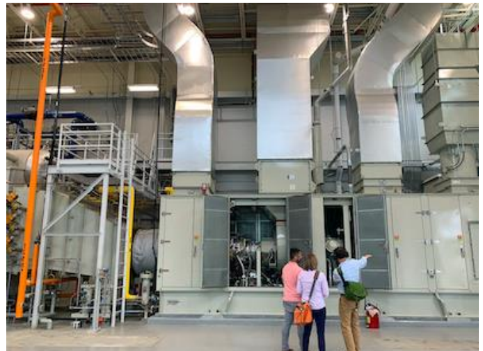
Erik Hall (far right), describes the CHP configuration including the combustion turbine at the Centennial Campus Utility Plant.
