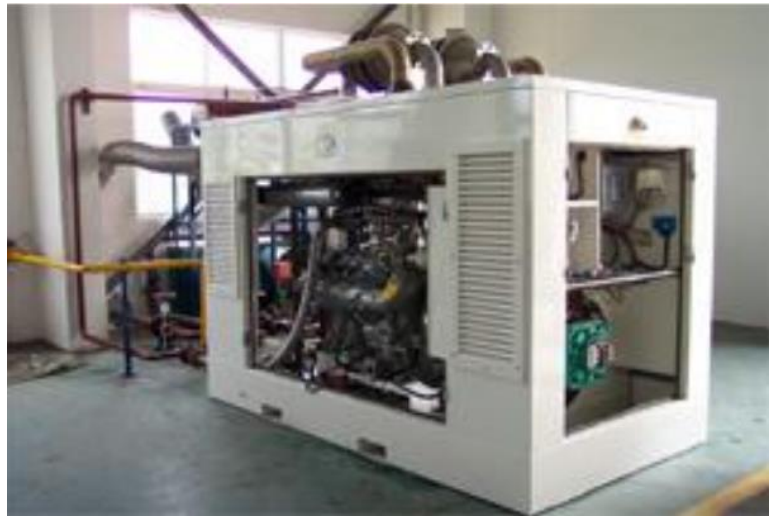
Stowell Distributed Power CHP Unit
