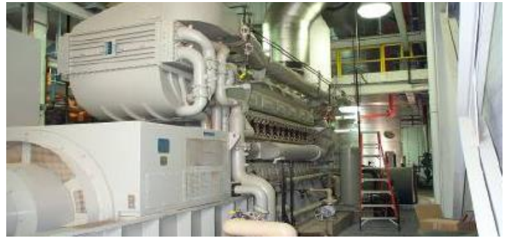
Fairbanks-Morse 3.2 MW dual-fuel generator
